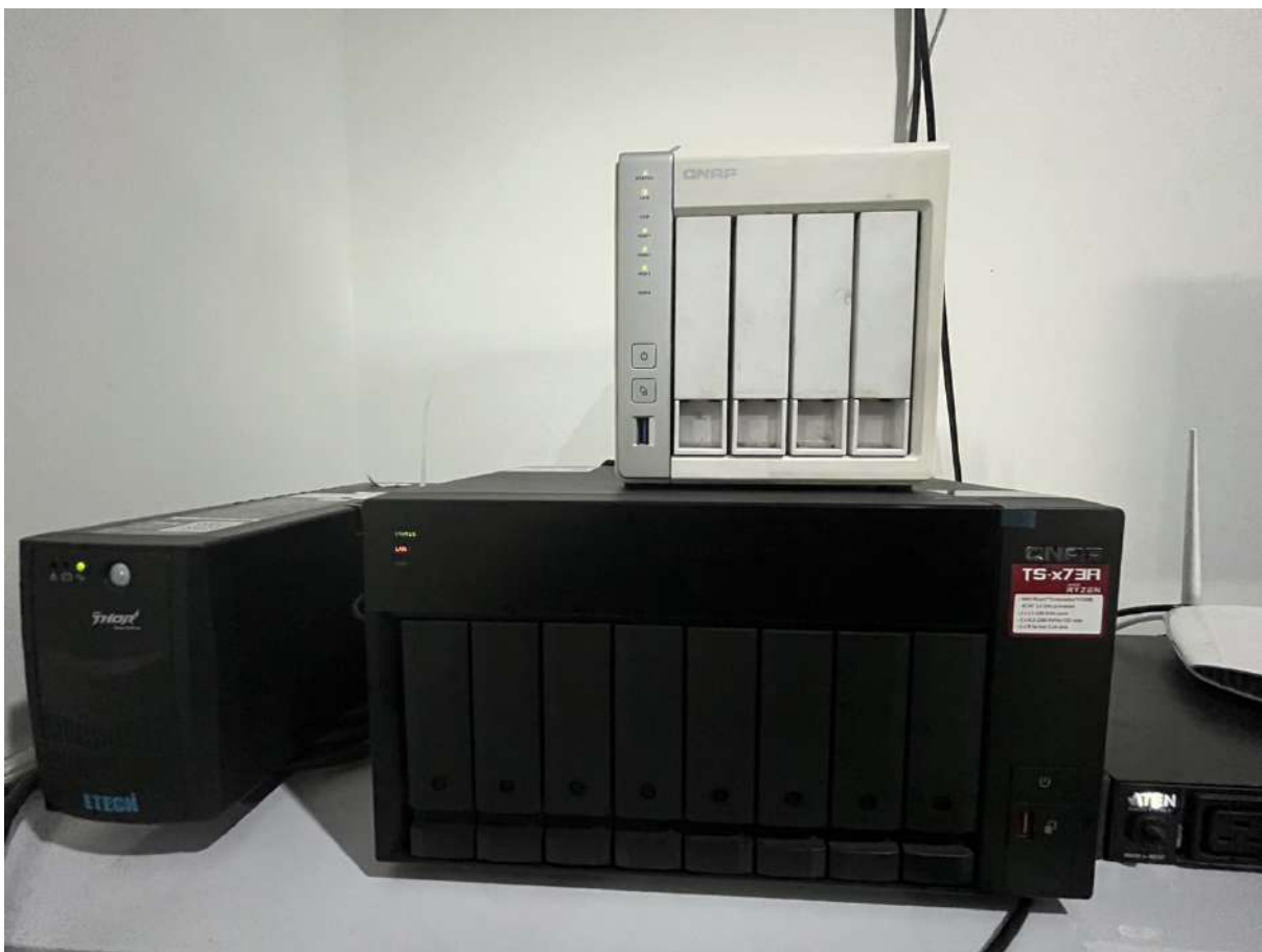
Qnap NAS Storage 32 TB
